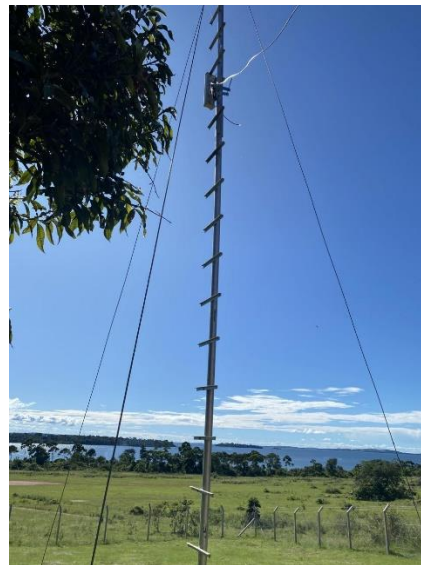
Figure 4: Sector Out Door Unit (ODU) Installed serving Bufumira HC III
